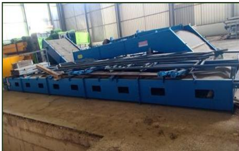
Figure 3. Image of Conveyor System in Waste Sorting Facility
