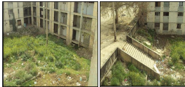
Figure 5. Condition of Exterior Spaces (Common Parts) of Martyrs Neighbourhood Buildings
