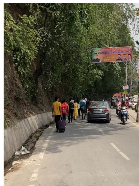
(Fig 2) Decrepit Retaining Wall
