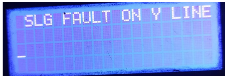
Figure 8.LCD display showing fault details of SLG fault
